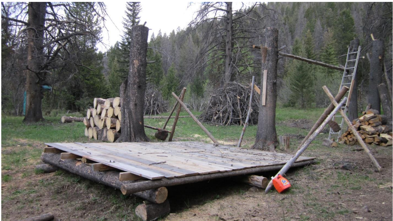
Figure E20. Tent floors built with dimensional lumber, supported by tops of large trees cut off leaving 10' stumps.
