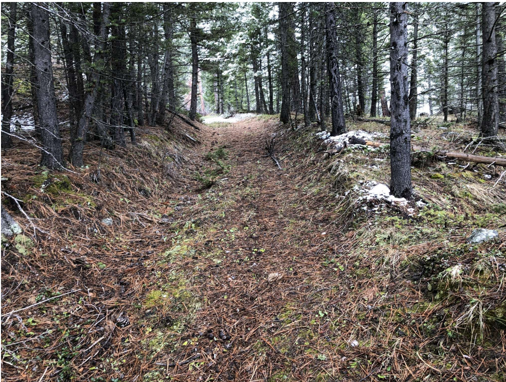
Waypoint 117 Looking up old, eroded, but now duff and vegetation covered road bed. S aspect.
