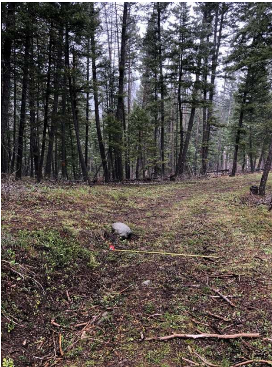
647-NS15-2 Looking north. Road cleared of blowdown.
